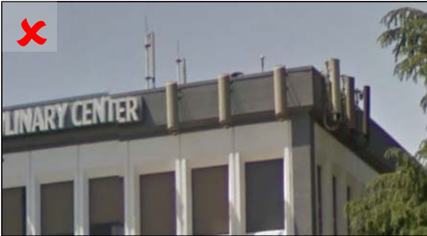
Figure 9 – Unsuccessful example of façade mounted equipment.
